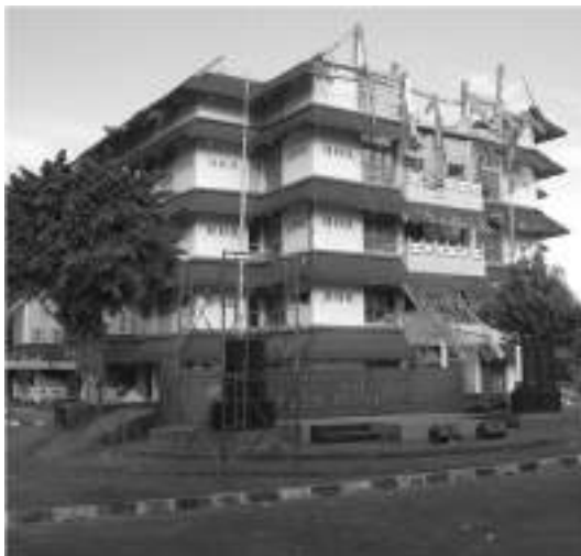
1 st Building → Collapsed Roof Structure
