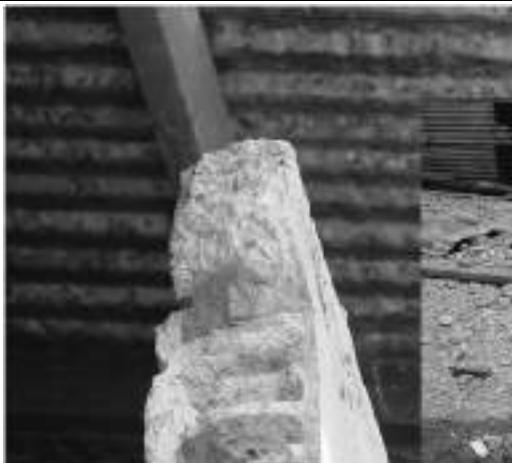
No steel inside concrete beam
