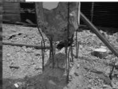
Very...very...small amount of confining steel inside concrete column
